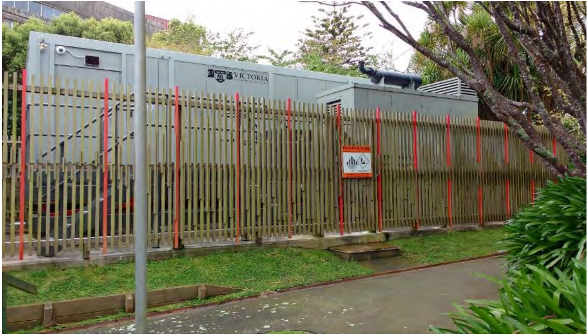
Photograph 5: View of the data centre with the independent generator and fuel storage.
