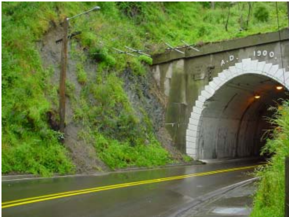
Figure 8 Crushed rock of the Wellington fault is exposed, at power pole, at the eastern portal of Karori tunnel (Photo: N.D. Perrin, Dec 2001).
