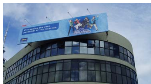
Signs should not obscure architectural features and should not project above the building roof top
