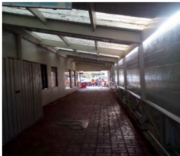
Lack of natural light
