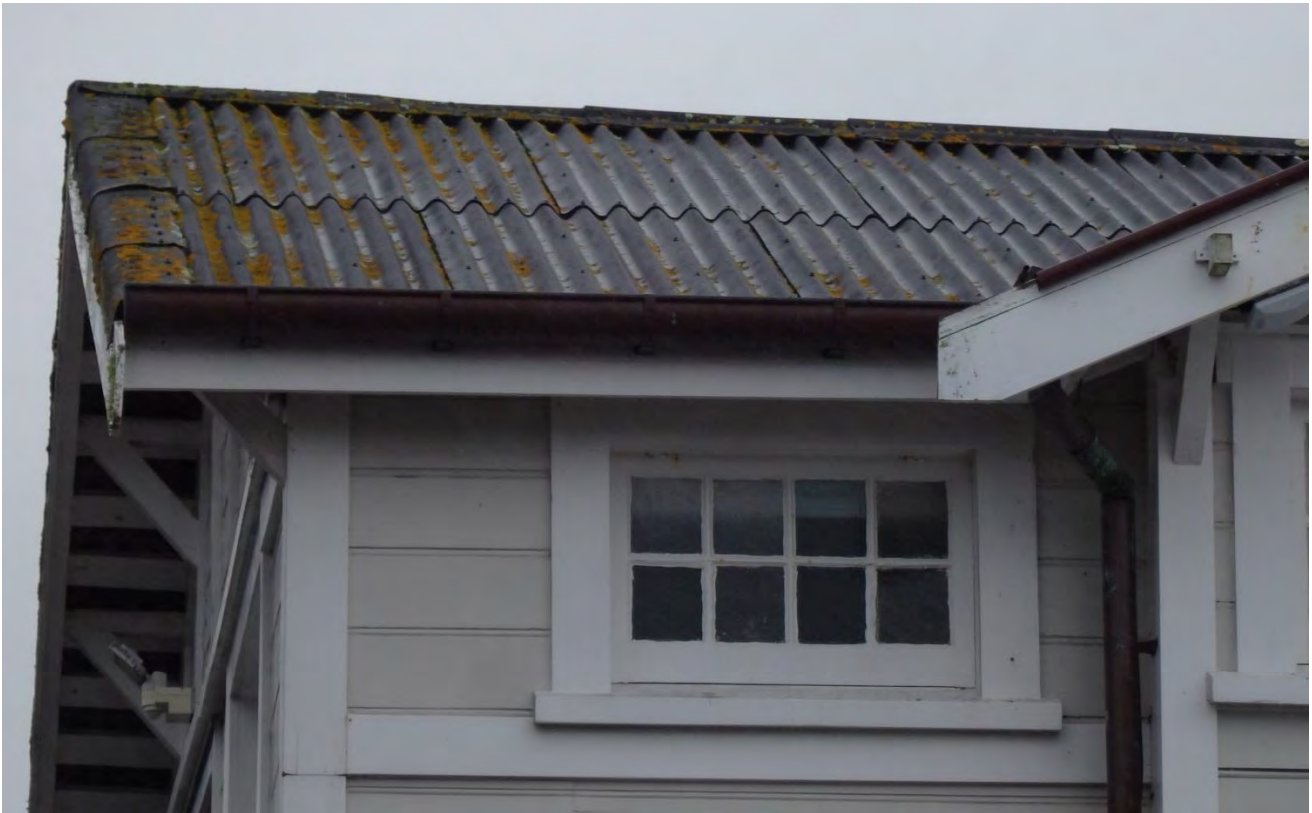
Khandallah Hall roof showing lichen build-up.
