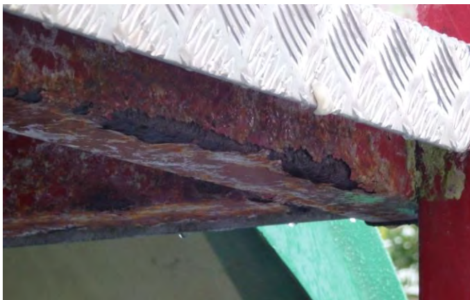
Rust under the playground structure at Khandallah library, 10th May 2018
