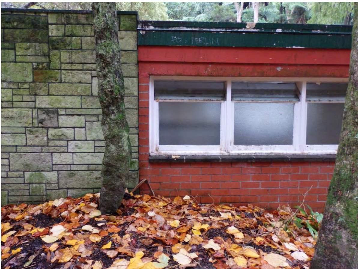
Khandallah pool building, 10 th May 2018. Note dirty peeling paint, moss, mould and mulch.
