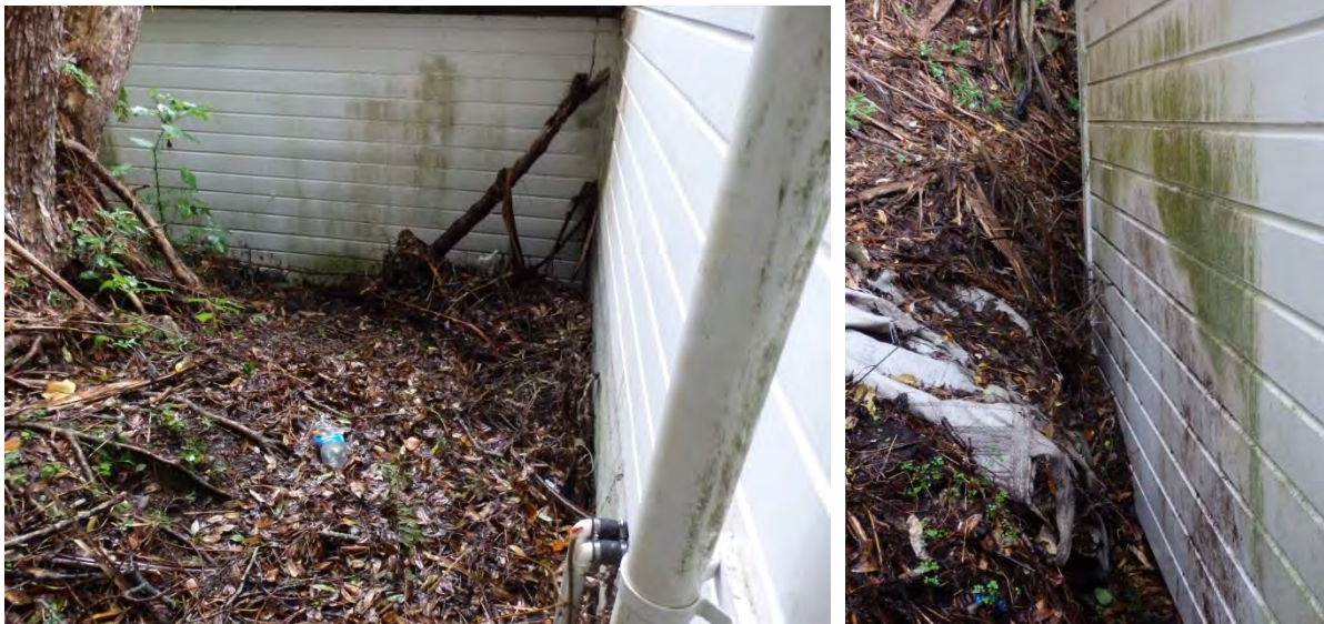
Khandallah Pool buildings. Note dirty mould walls and rubbish/leaf mould build-up. 10 th May 2018
