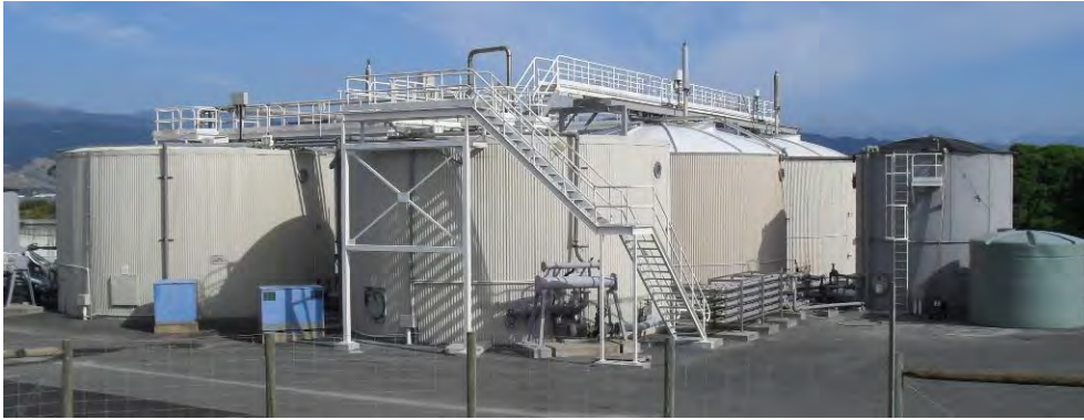
Figure 8: ATAD facility in Nelson, New Zealand
